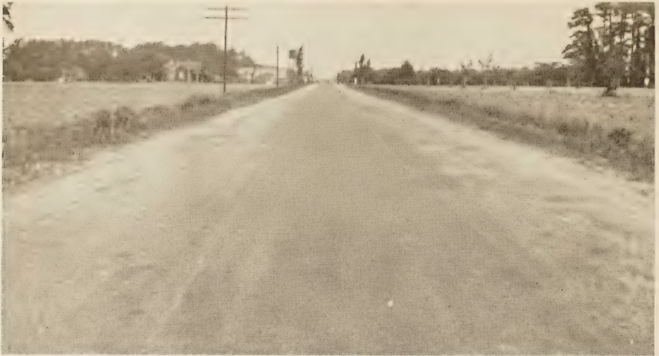
FIGURE 12.—VIEW OF EXPERIMENT 8 TAKEN 4 YEARS AFTER CONSTRUCTION. THIS IS TYPICAL OF THE APPEARANCE AND CONDITION IT HAS RETAINED SINCE CONSTRUCTION.
